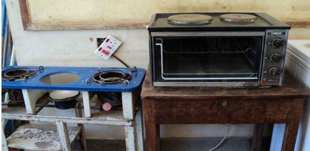
Photograph 3: Damaged Cookers in School 'C'
