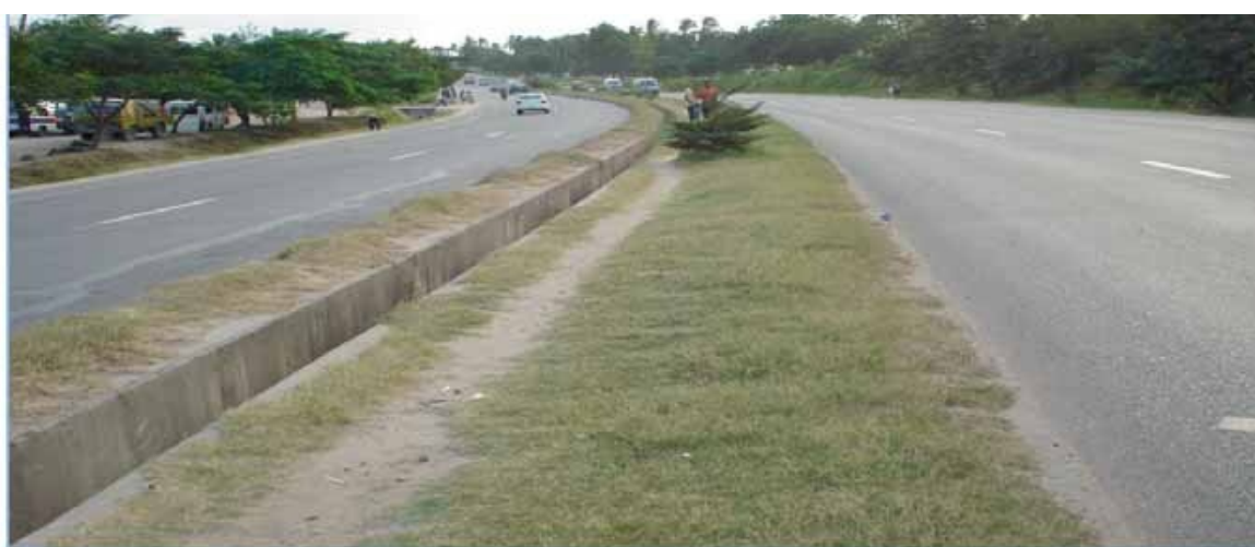
Figure 1: Missing Warning signs at the end of dual carriageway (End of dual carriageway – Kimara).
